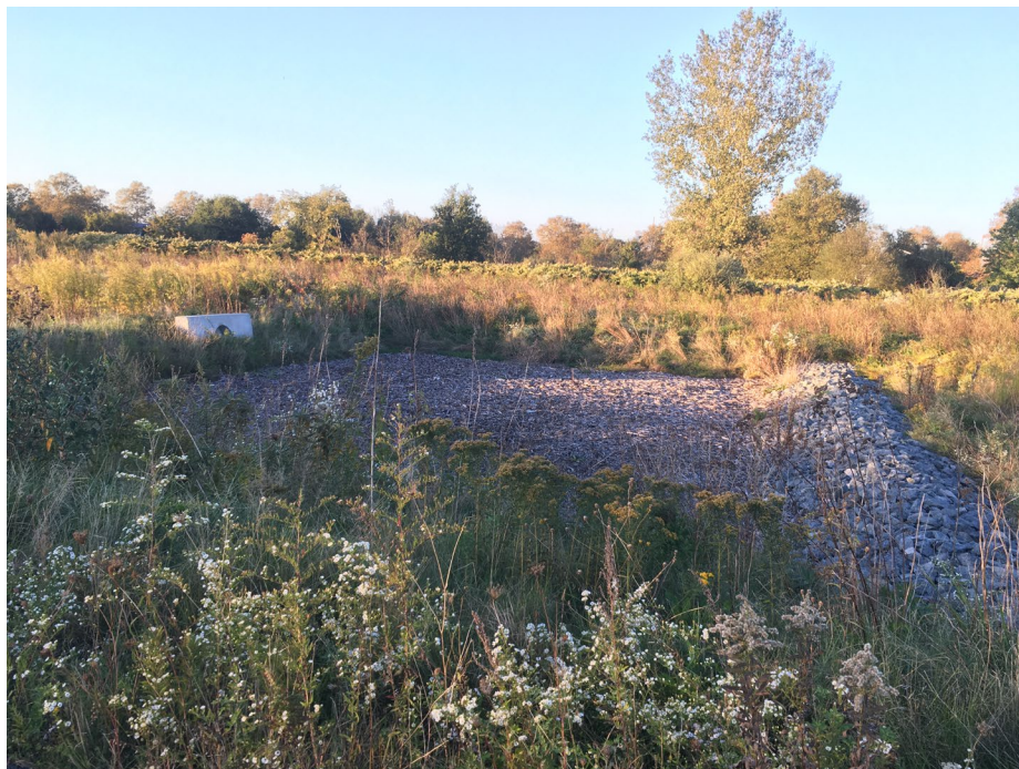
Photo 4: View of the incomplete stormwater feature along the access drive facing north.
