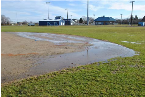
Drainage issues at Gaudet
