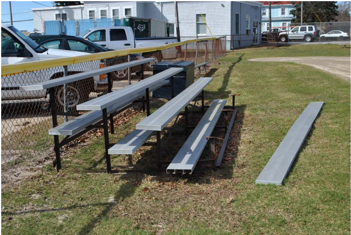
Bleachers at Oliphant are in disrepair
