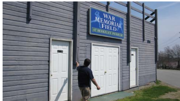
Bleachers are in poor condition
