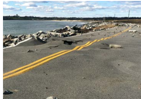
Sachuest Point Road after Hurricane Sandy, October 2012
