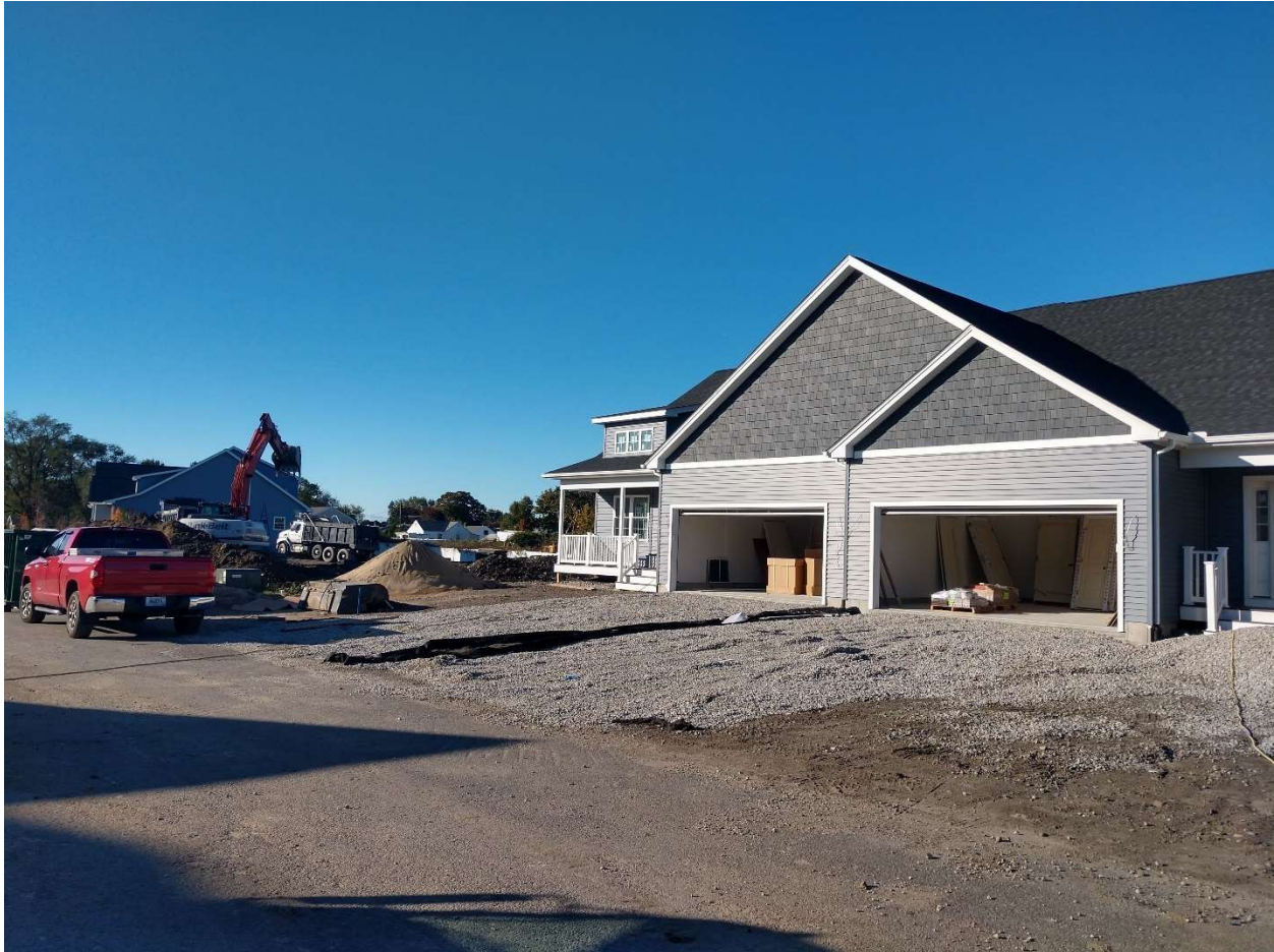
Figure 2.7 Photo of Senior Living Community Construction off of West Main Road, October 18, 2019
