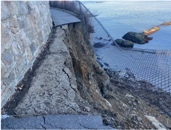
Erosion of the Cliff Walk in March 2022.
