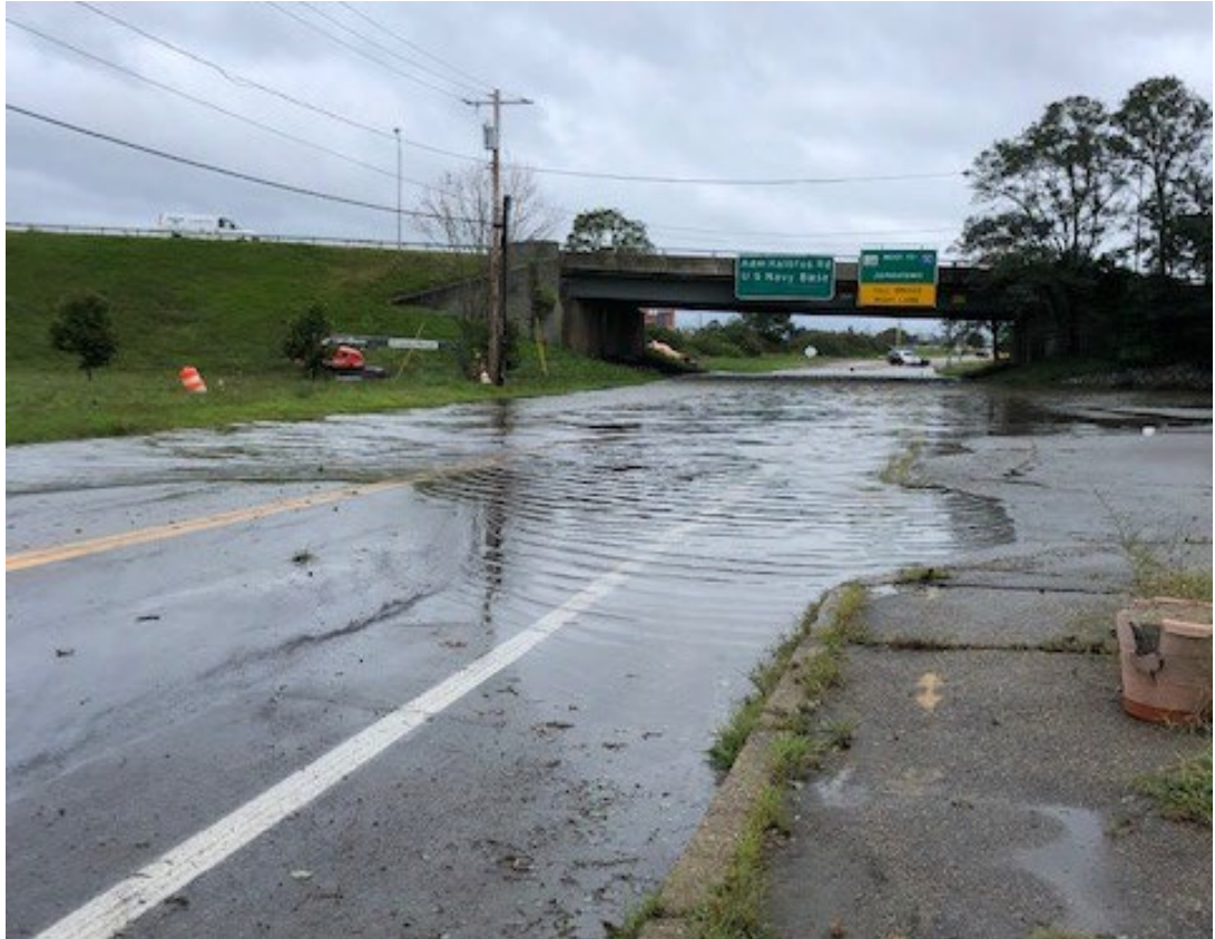
Flooding at JT Connell Highway on Sept 2, 2021 after the remnants of Hurricane Ida.
