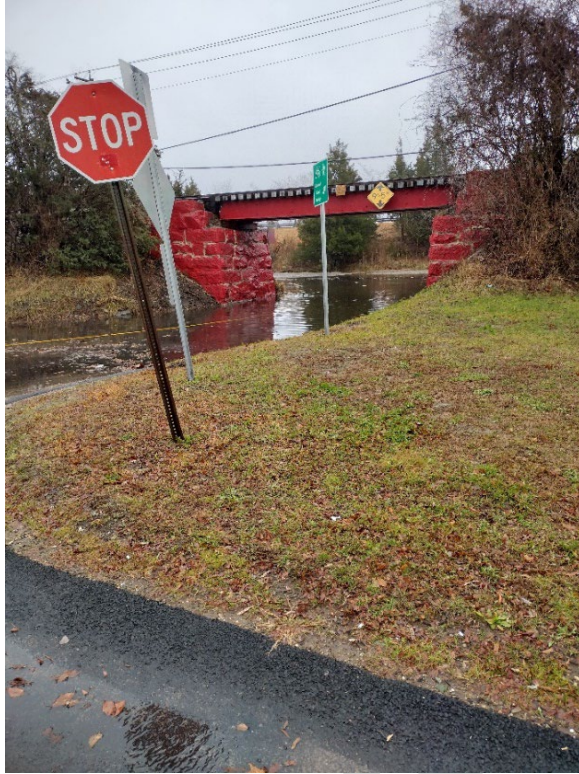
Road flooding at entrance to Common Fence Point, Portsmouth. Grant money was used to install a better drainage system reducing the flooding depicted above but concern now exists as tides creep higher and water egresses in from the drainage system during extreme hightide events.
