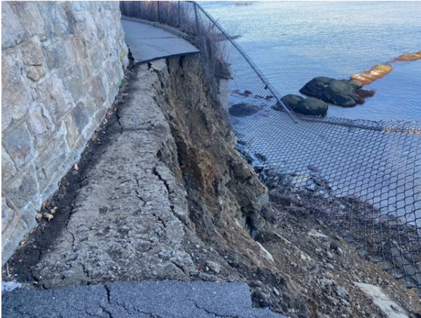
Erosion of the Cliff Walk in March 2022.
